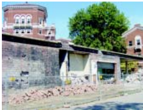
The Weatherford Hall dining center has been demolished to make room for a grass amphitheater.
